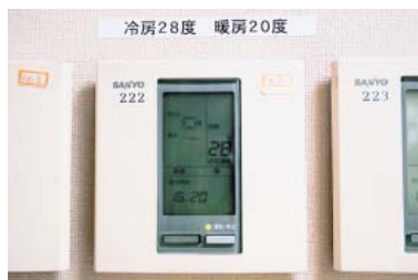
Controlling air conditioner temperature
