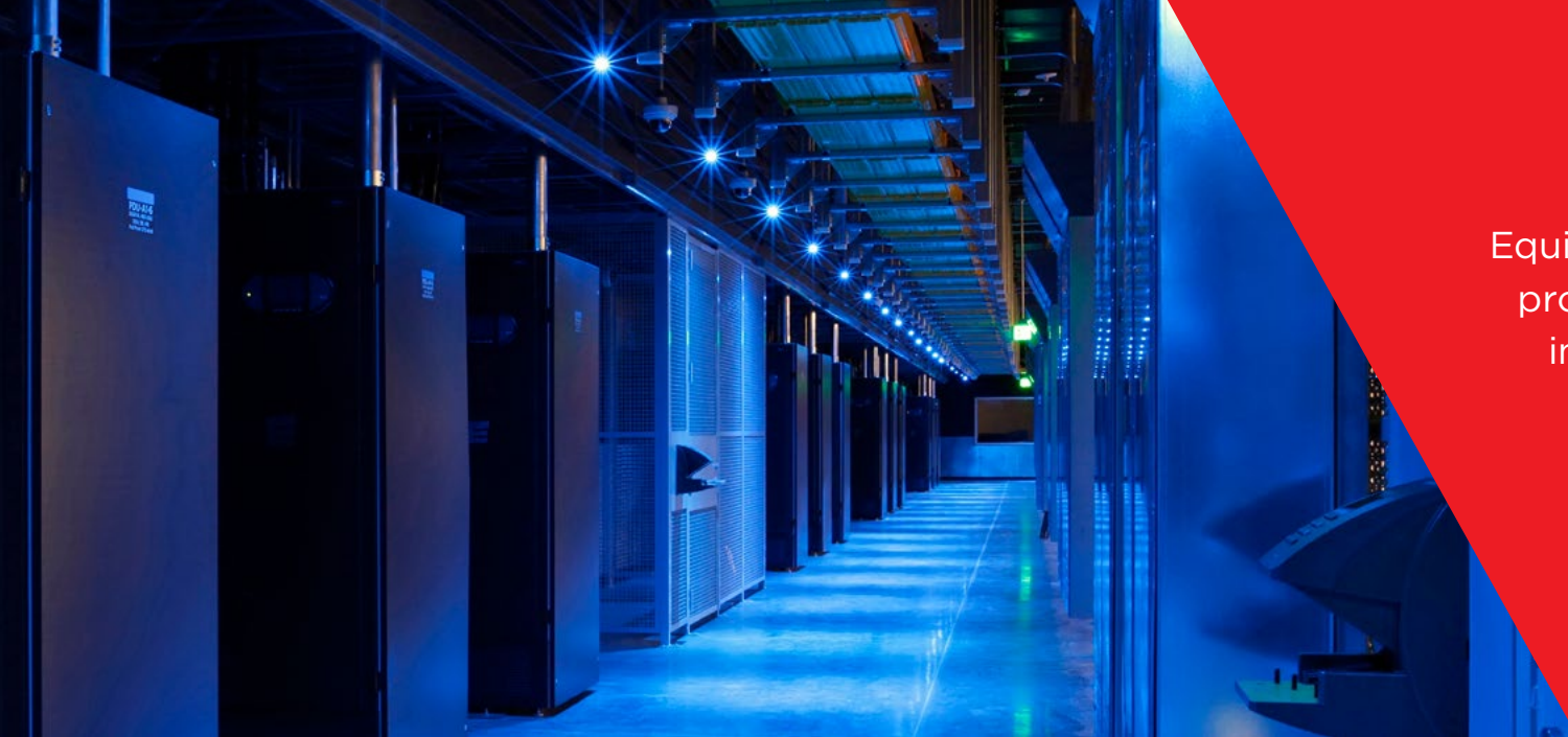
SV10 Silicon Valley IBX® Data Center
