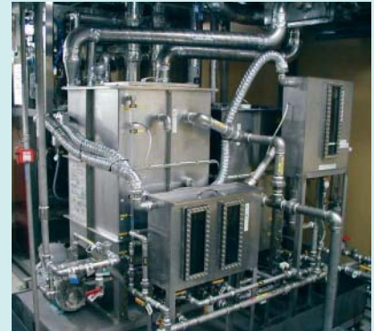
Photo 1 New butyl acetate recycling machine at the Hirooka Plant
