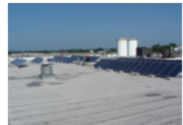
American Flange reduced their electric consumption by 10 percent with solar panels.
