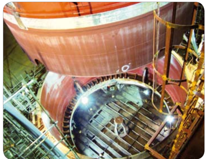
Top Construction of our new production facilities in Asia Bottom Turret shaft at our Chim Sáo drilling operations, Vietnam
