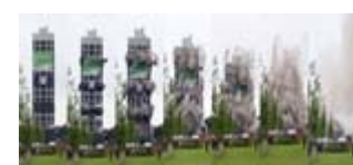
Fig 17– Bannerbrook Park, Coventry tower demolition where concrete rubble has been recycled and reused
