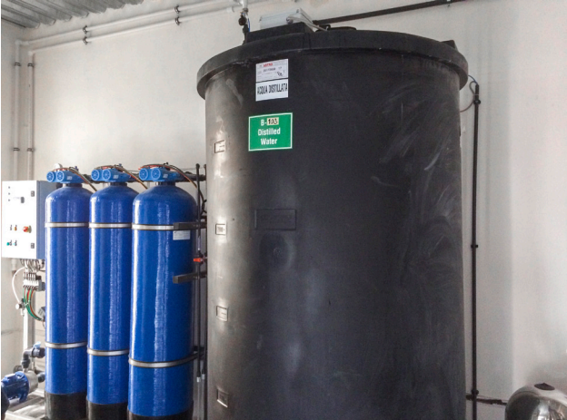
In Uzbekistan, the new wastewater treatment plant guarantees water reclamation of 90 to 95%.
