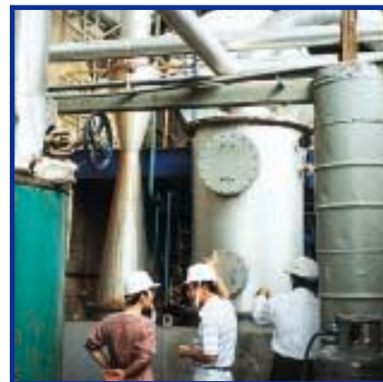
The Environmental Office and Sony Video Taiwan conduct a risk assessment exercise at the facilities of a waste treatment contractor.
