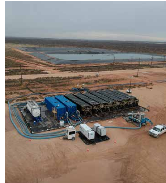
TETRA water treatment and recycling facility.
