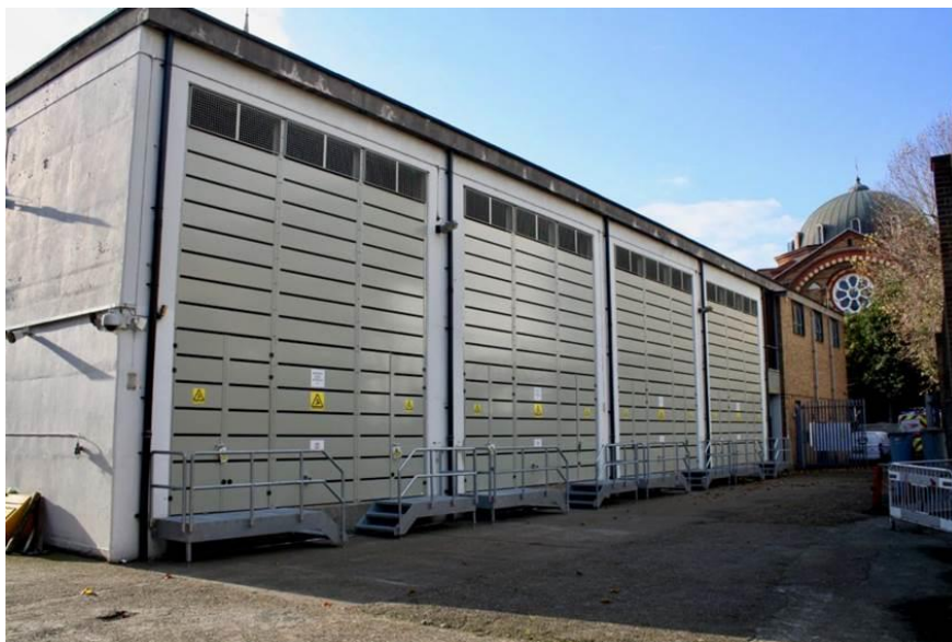
Figure 7: An innovative noise screen installation at a substation in our LPN region
