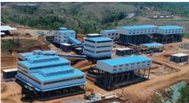
Figure 3. Wilton's 500 tonnes per day Flotation and Carbon-in-Leach mineral processing plant in Ciemas
